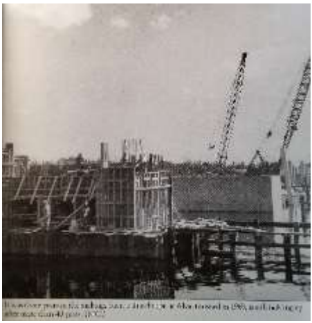
After the NASA missile barge hit the second swing bridge, the present bridge was built
